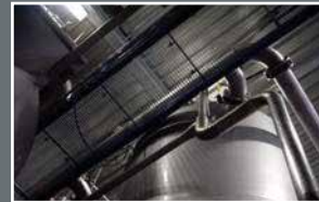
Advanced treatment Physico-chemical treatment
